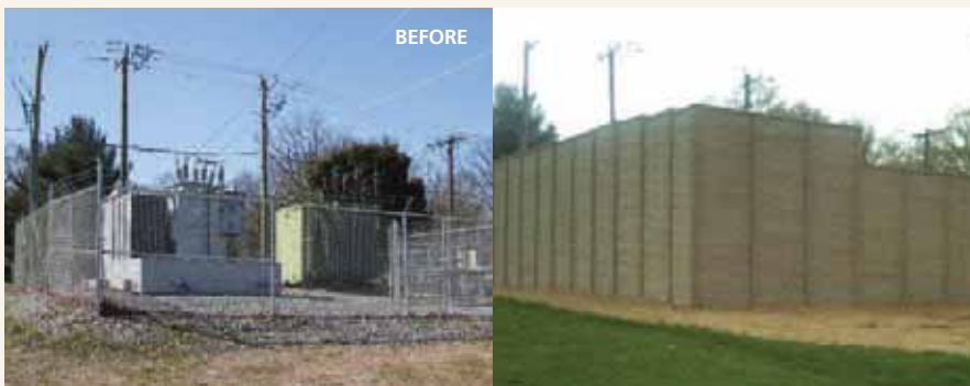
A newly constructed enclosure makes this substation a quieter and more attractive 'neighbor.'
